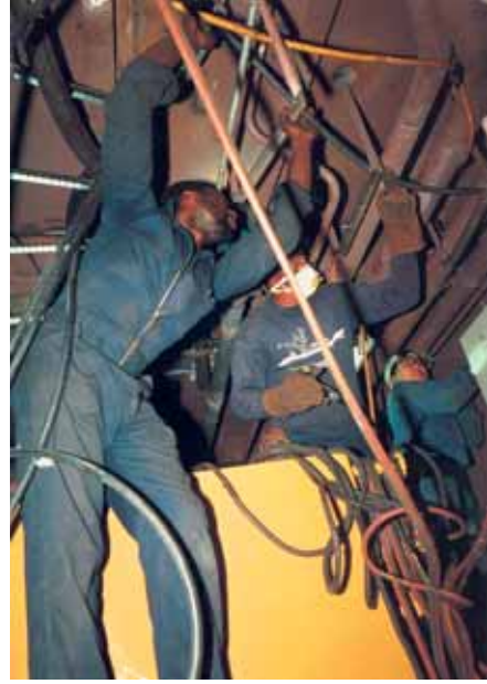
2b Pipe fitters finishing the engine room of a tuna-fishing boat. Campbell Shipyard. San Diego harbor. August 1991. (in: Sekula, S. 15.)
